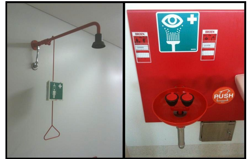
Eyewash stations are located in Building 8360, 8361, 8370
